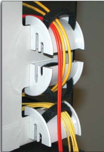
Patch Panel Egress
